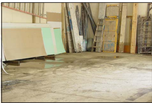
(Painesville, OH) This warehouse/storage garage shows extensive flood water damage after more than nine inches of rain fell, July 27. Joint damage assessment teams conducted surveys of infrastructure damage in Ashtabula, Geauga, Lake and Cuyahoga counties this week. (Ohio EMA photo by Vikki Bunting).
