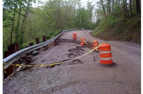
April/May 2011 flooding southern Ohio.
